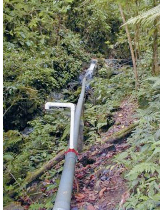
This PVC penstock routes the water from the small dam down the hill to the turbine where it generates electricity.
