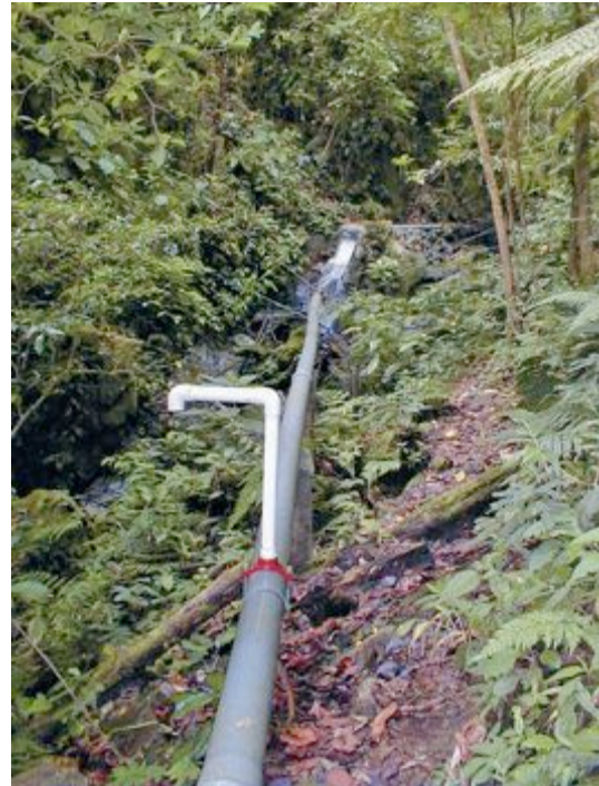
This PVC penstock routes the water from the small dam down the hill to the turbine where it generates electricity.
